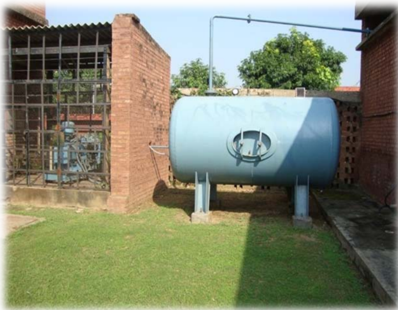
Compressed Air Vessel
